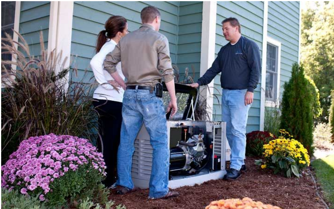
Figure 4. A 22-kW gas-fired standby generator. A 20-kW cold fusion generator will be about this size, and will produce up to 14,600 kWh/month (Lowe's, Inc.)
