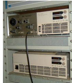
Fig. 7: Photo of power supply
